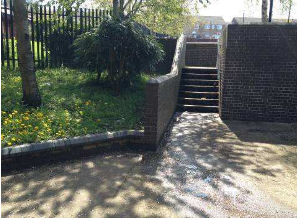
Footpath (Point (A)) subject of stopping up request - set of steps at the northern end into the car park
